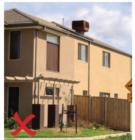
This cooling unit is visible from the primary and secondary streets, and so does not comply.
